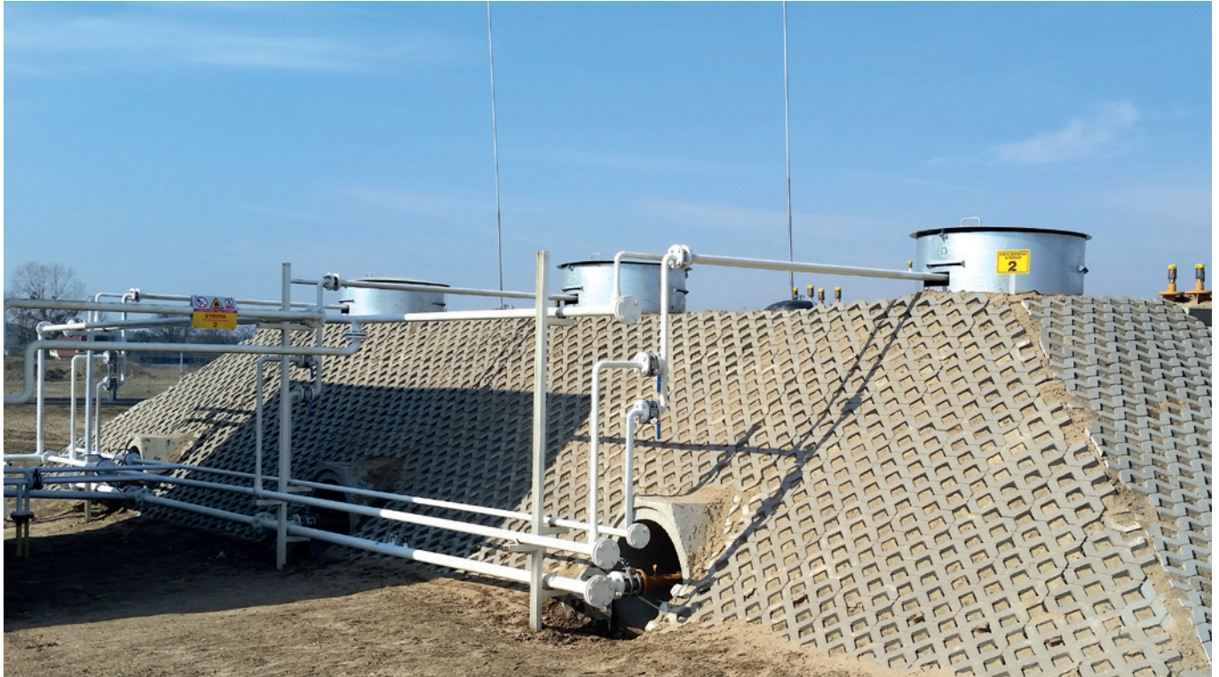
Project LPG Distribution Facility: 3 x 50 m 3 , Ø 2500 mm
